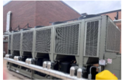
FIGURE . OUTDOOR UNIT OF AIR TO WATER HEAT PUMP SYSTEM
