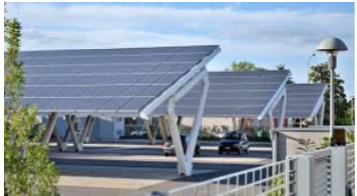
FIGURE . CARPORT SOLAR FROM GREENLANCER.COM
